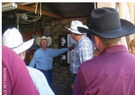
Here, Dennis Moroney explains the use of a solar inverter during the workshop.
